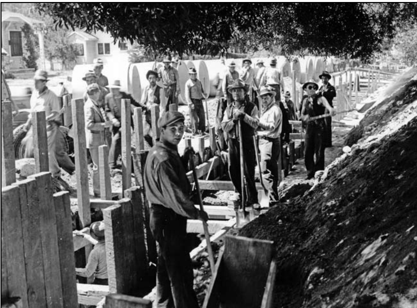
1938 WPA workers labor on a lateral drain on Avoca Street. (photo courtesy of USC Library, CHS collection)
