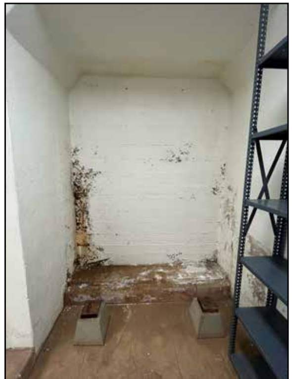
Katie Taylor's sharp eye and our online camera revealed that the leakage was coming through the south wall of the closet, the walled off historic entrance to the 1914 Library basement. This photo shows the damage to this wall revealed when our materials were removed to storage. (Photo by Katie Taylor-ERVHS)
